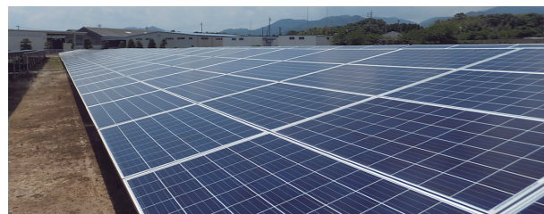
Solar power generators (Nichino Service Saga Plant)
