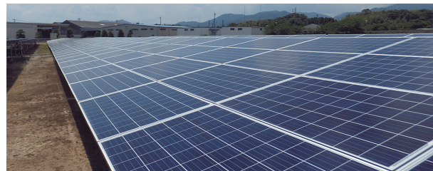
Solar power generators (Nichino Service Saga Plant)
